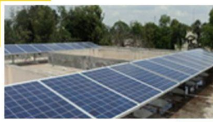
ROOF TOP SOLAR SOLUTIONS
